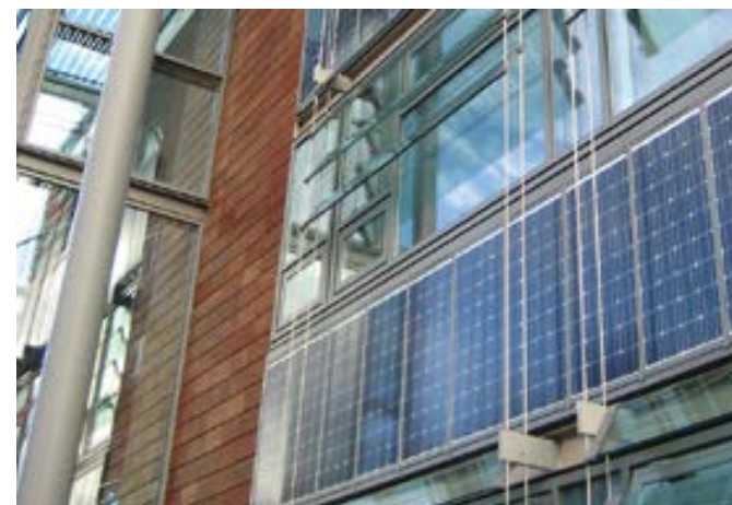
Integrating micro renewables—Kings Buildings Solar Panels are integrated into the design of the elevation.
